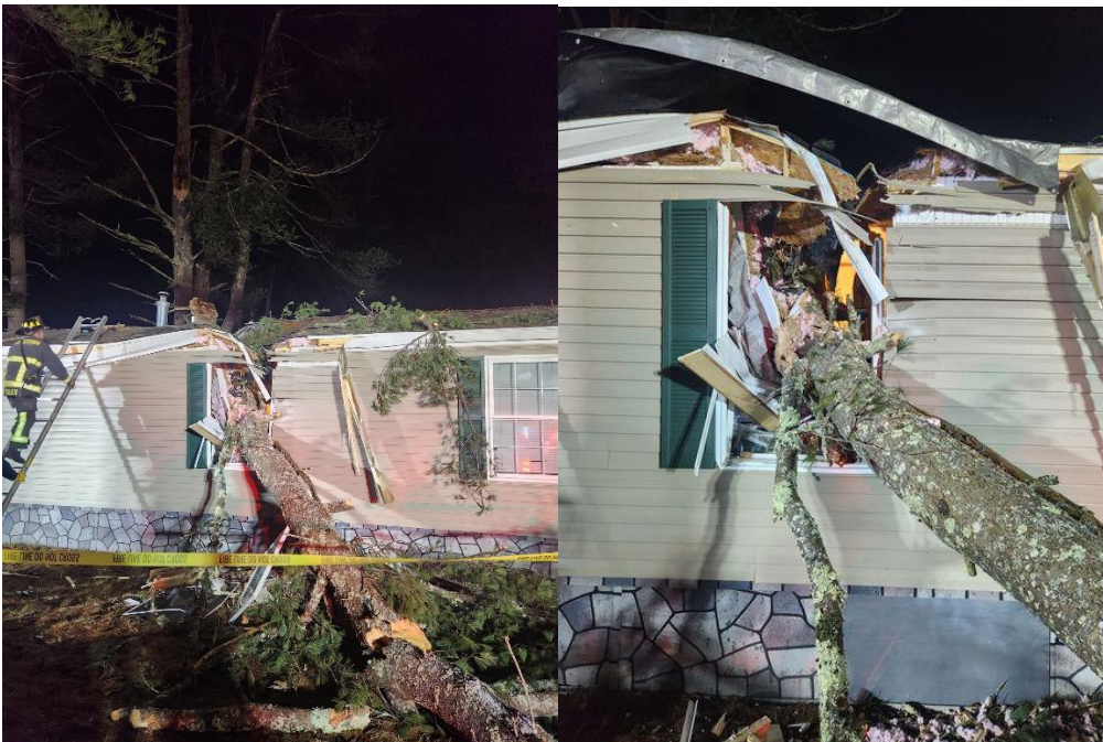
Crews from New Boston and Goffstown responded to a tree into a building on Parker Road. Luckily no one was injured. Crews secured all utilities and tarped the structure to prevent further damage.
